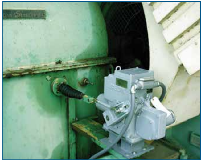
Raw Mill Dust Collector Fan Speed Control
