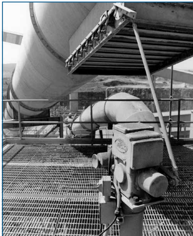
Baghouse Tempering Air Damper
