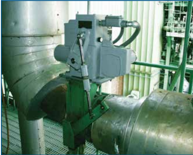
Main Fuel Gas Valve
