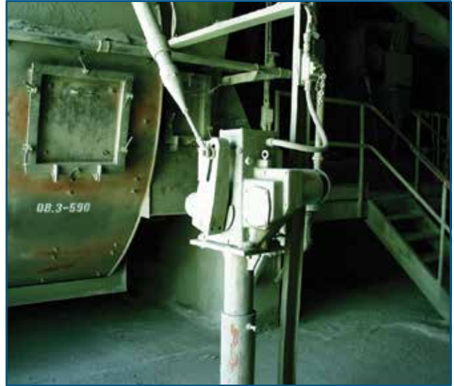
Primary Air Fan Damper
