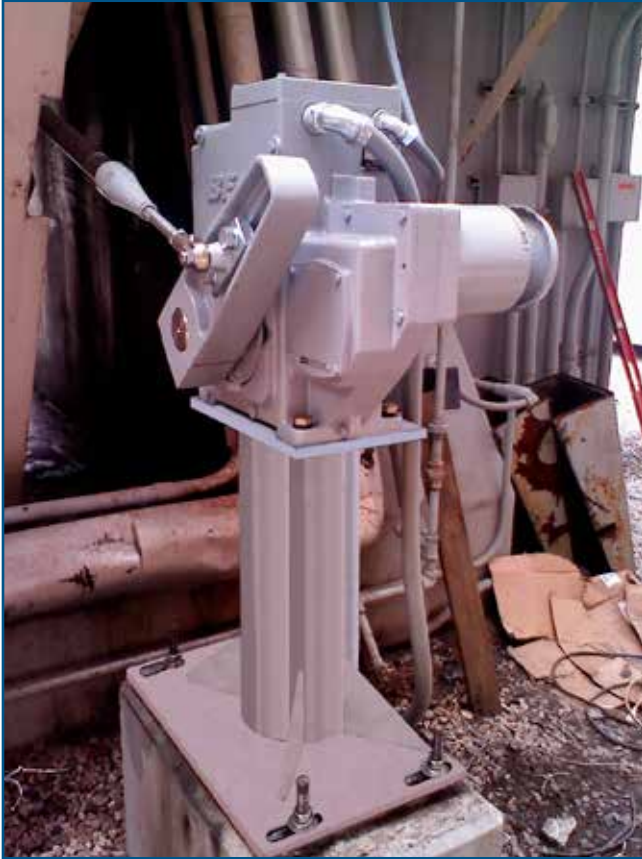
Beck replacement installed on an ID fan damper. Note obsolete pneumatic line.
