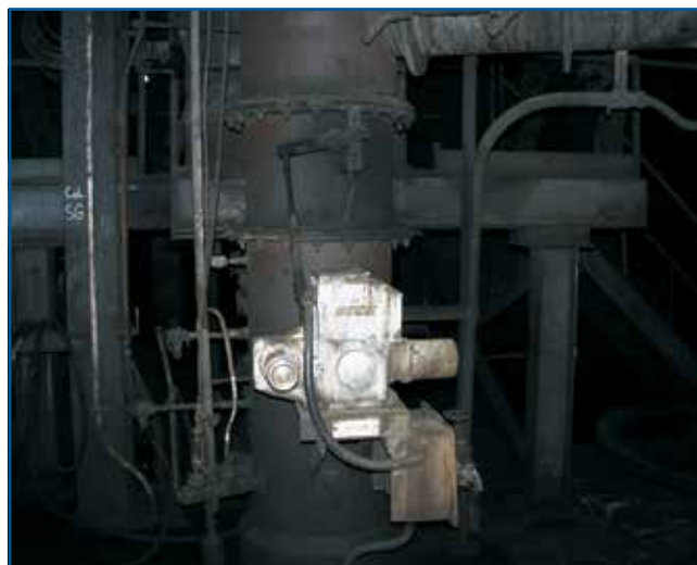
Beck actuator installed on a coal mill exhaust damper.
