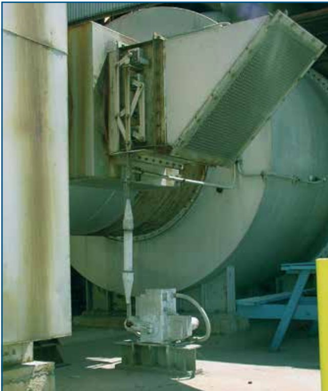
Model 11-200 on a Mixing Air Damper
