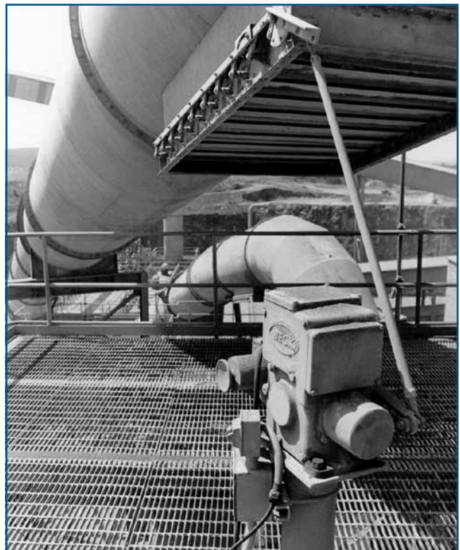
Baghouse Tempering Air Damper
