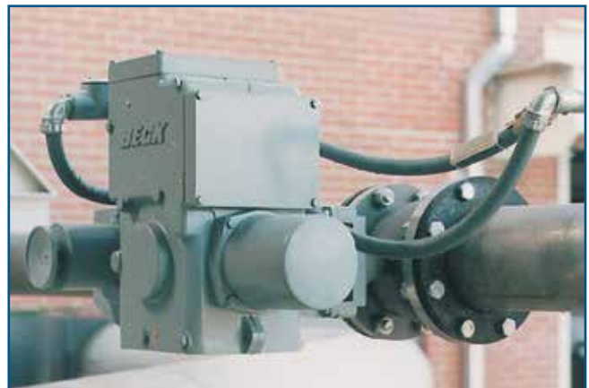
Refiner pressure control valve
