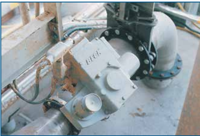
Machine chest recirculation control valve
