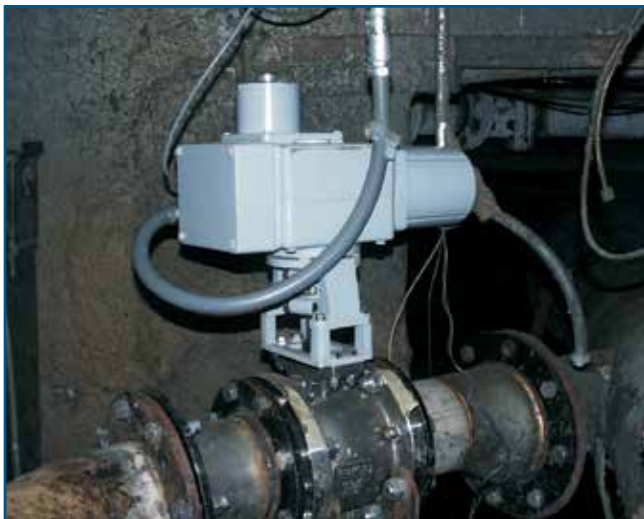
Vat level control valve
