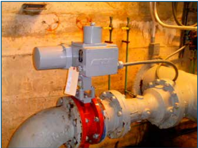
Beck actuator installed on a filter effluent valve
