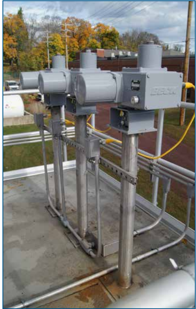
Beck Model 11-160s mounted on sludge valve extension bonnets
