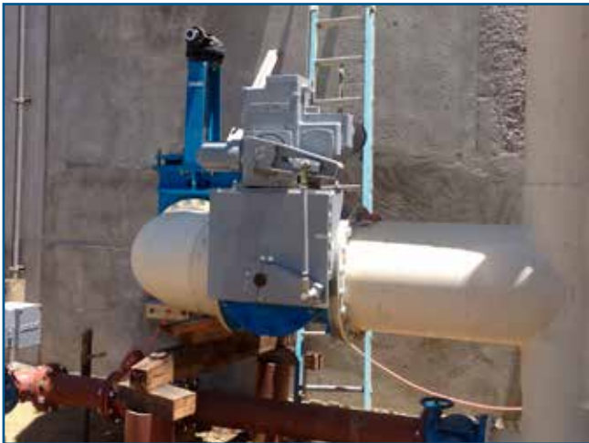
Beck actuator installed on a digester valve in a hazardous-rated application
