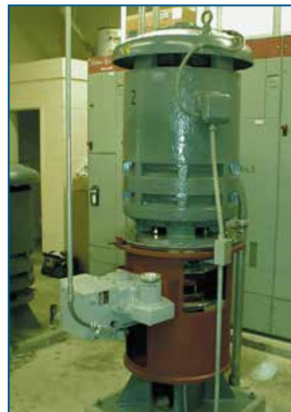
Beck Model 11-200/300 installed on a MagnaDrive Vertical ASD
