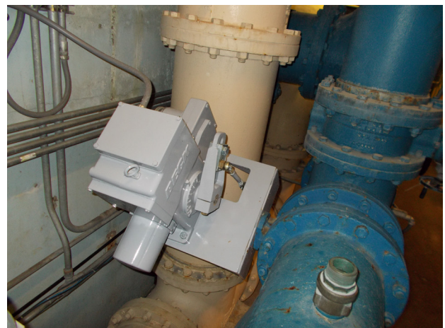
Figure 5 - BECK actuator on Filter Effluent Valve
